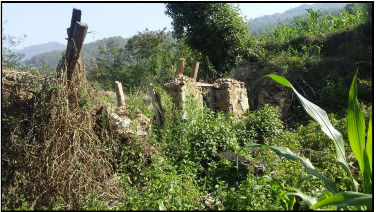
Figure: 1 Earthquake damaged households at downhill of Tallo Mati
