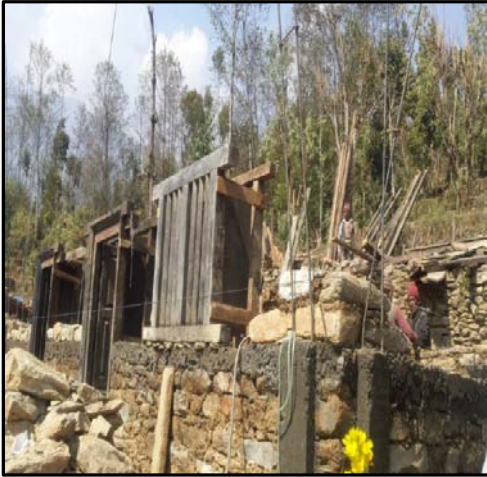
Picture 2: House under construction with optimal use of salvaged materials at BadhuwaSimtoleSundrawati
